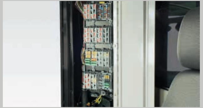
The electric fuses panel.
